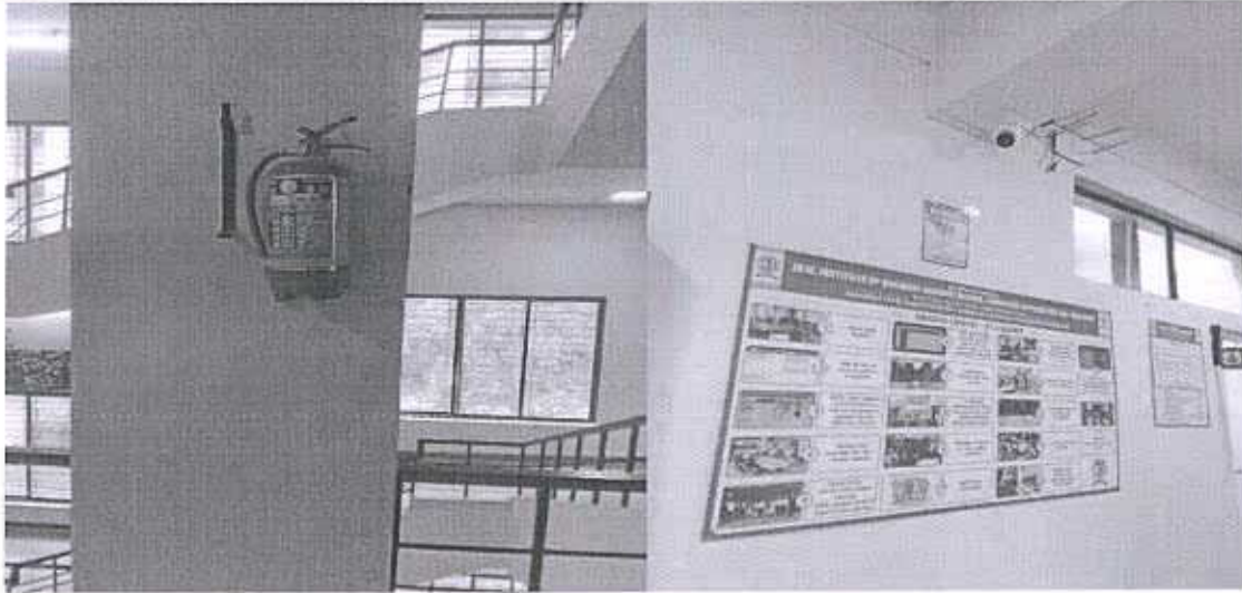
Safety Measures : Fire Extinguisher and CCTV
