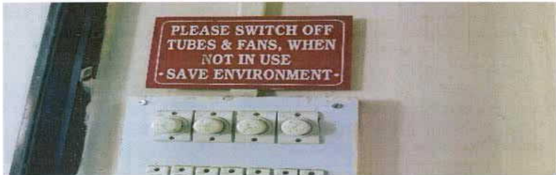
Typical display board near each switch board
