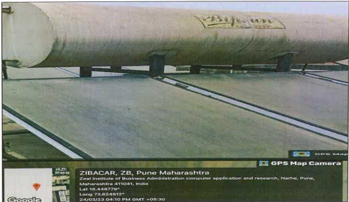
Solar panels at rooftop
