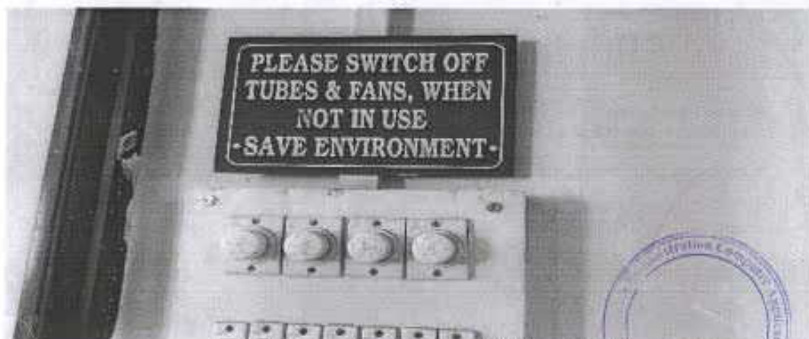
Picture of note near switch board
