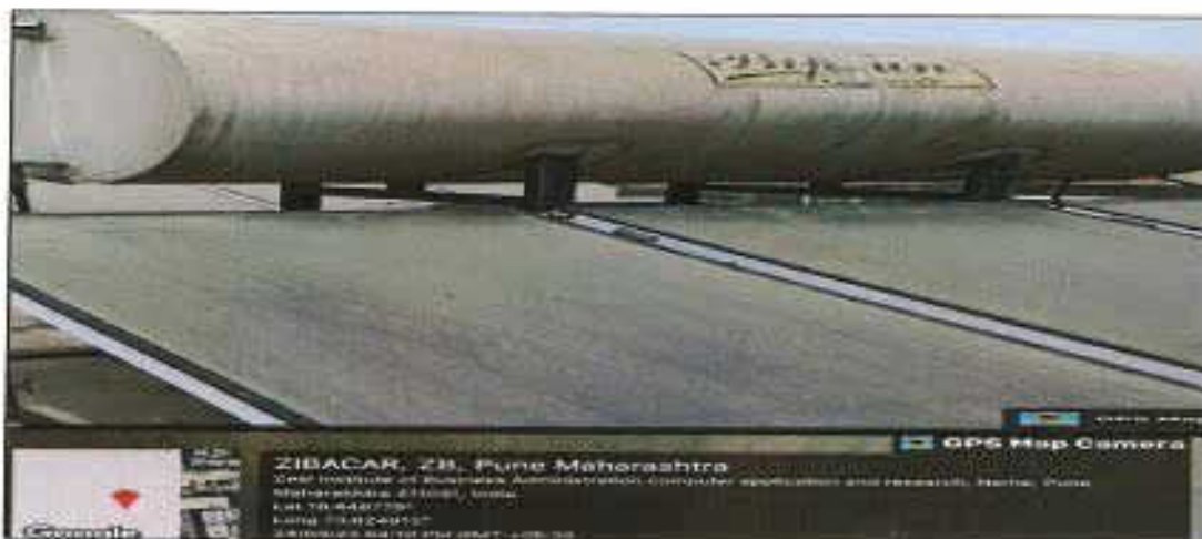
Solar panels at rooftop
