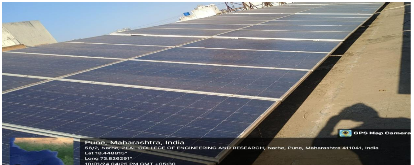
Solar panels at rooftop
