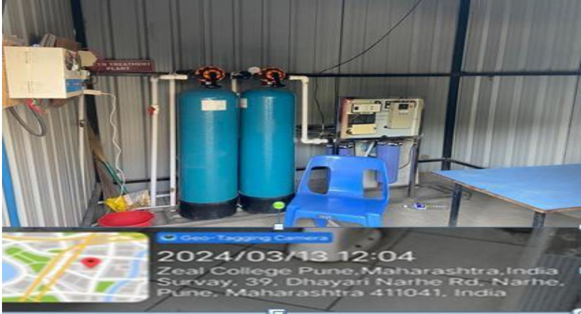
Image-7.1.4 (4a) - Water recycling and Filtration @ ZES Campus
