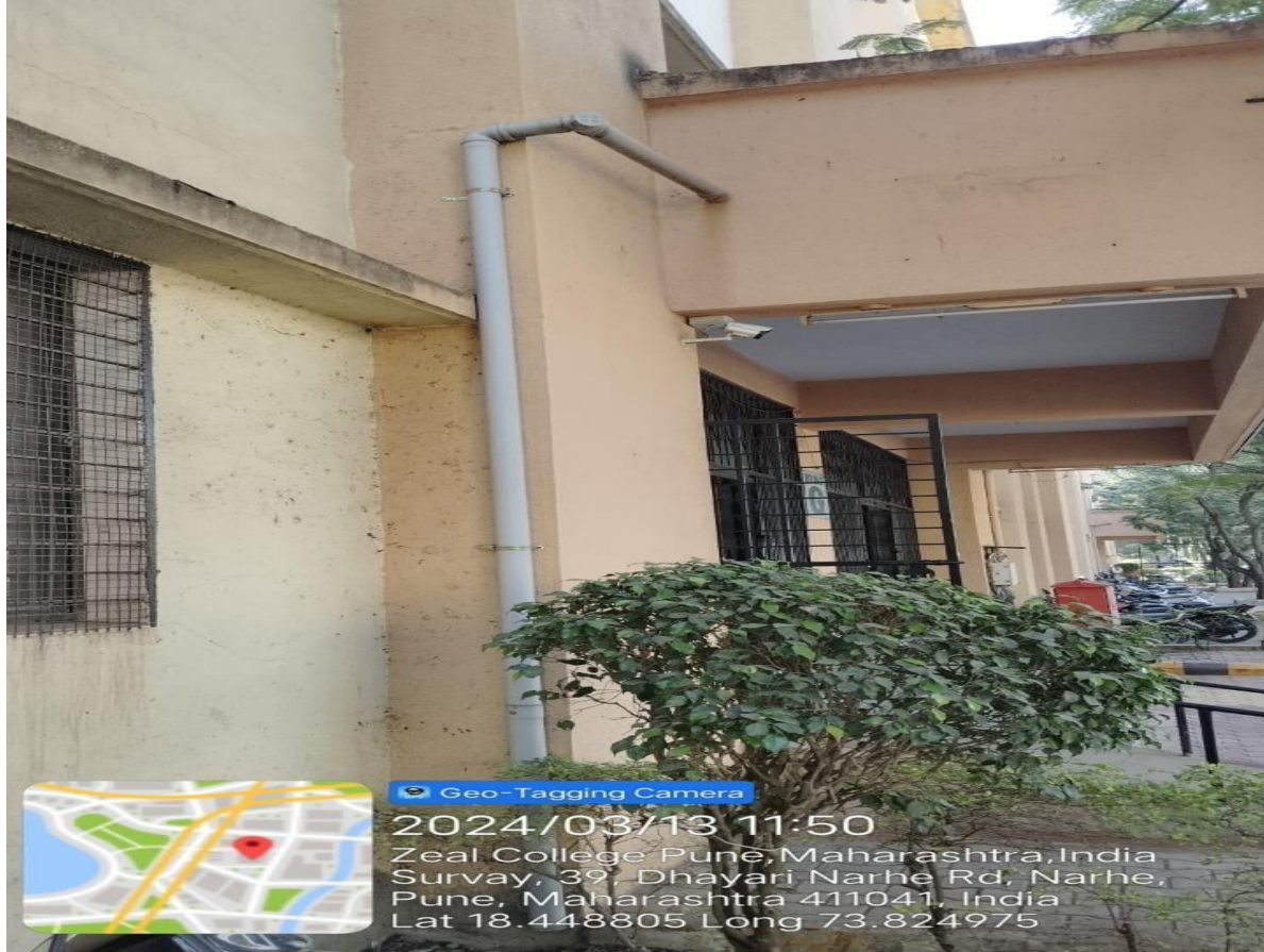
Image-7.1.4 (1b) -Rain Water Harvesting System
