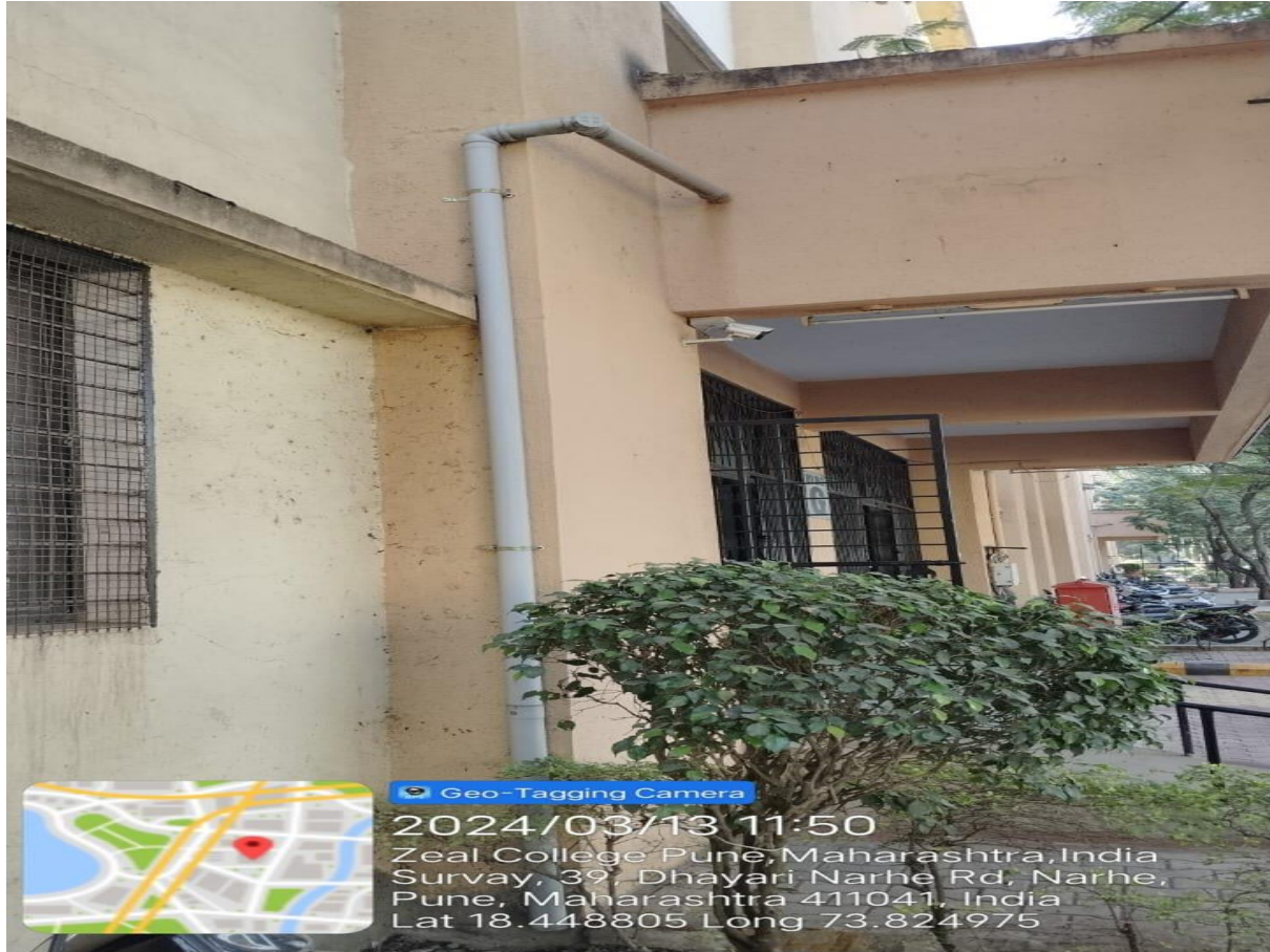
Image-7.1.4 (1b) -Rain Water Harvesting System
