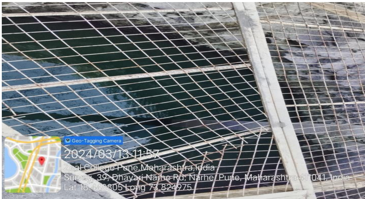
Image-7.1.4 (2a)-Open Well Recharge System @ ZES Campus
