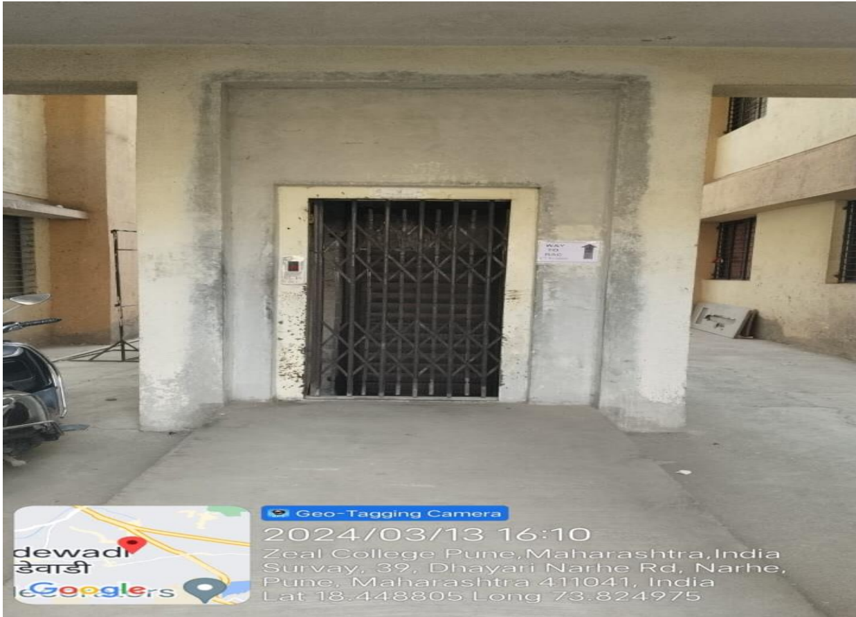
Image-7.1.7.2(e) Lift made available for ease of access at entry point ZIBACAR
